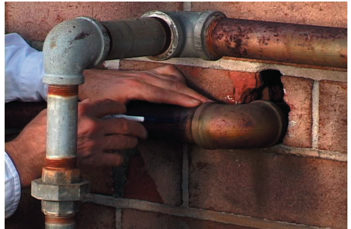
Figure 3. The places where utility services penetrate the façade of the building provide a perfect entrance for pests. Be sure to inspect the exterior of your facility with a pest management provider and your onsite maintenance team to identify locations that need sealing or repairs to prevent pests from slipping inside.
